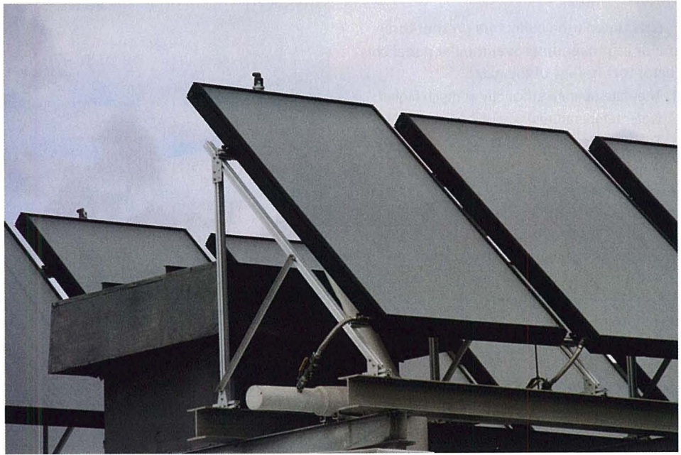
Figure 2 Flat panel array
